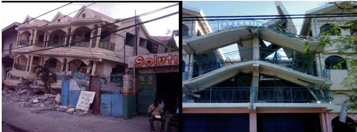
Fig. 1: Affected buildings in Port-au-prince
